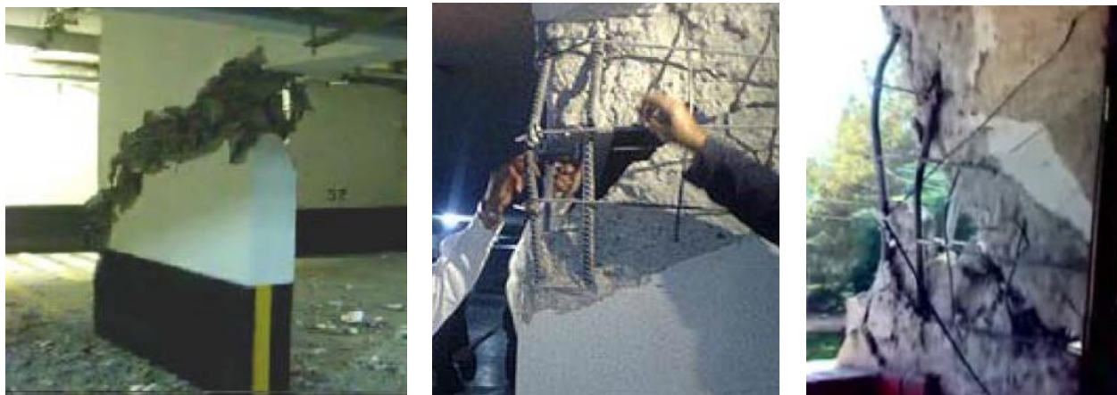
Figure 2.1 – Structural damage during Chile 2010 earthquake
