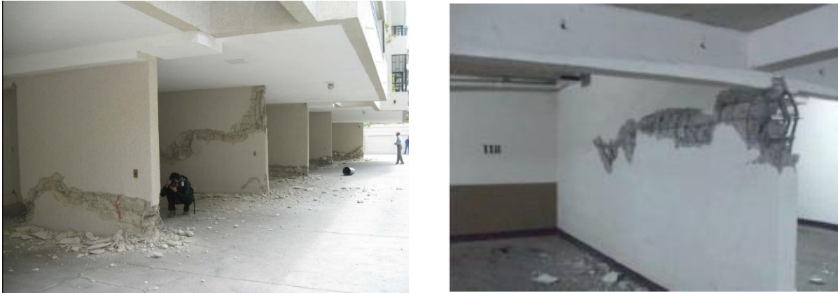
Figure 1-1-Flexural RC walls failure during Chilean (2010) earthquake. Source: adapted from San Bartolomé et al. (2011)
