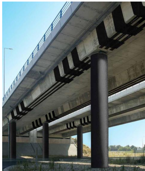
Figure 5. FRP reinforcing systems on bridges. Source: DocPlayer.
