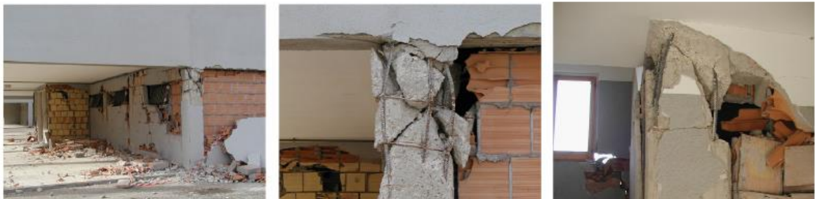
Tomado de Identification of the structural model and analysis of the global seismic Behaviour of a RC damaged building
