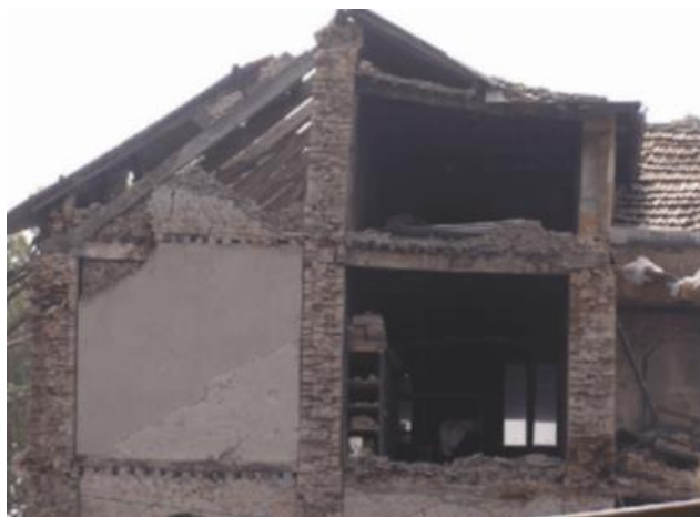
Figura 13. Colapso de cubierta en vivienda de mampostería. Nepal, 2015. Tomado de: Performance of Residential Buildings during the M 7.8 Gorkha (Nepal) Earthquake of 25 April 2015.
